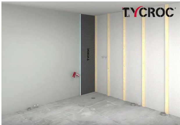
Before mounting the next board, Tycroc Premium Fix adhesive sealant should be applied to the edge of the previous board to glue the building boards to each other.
